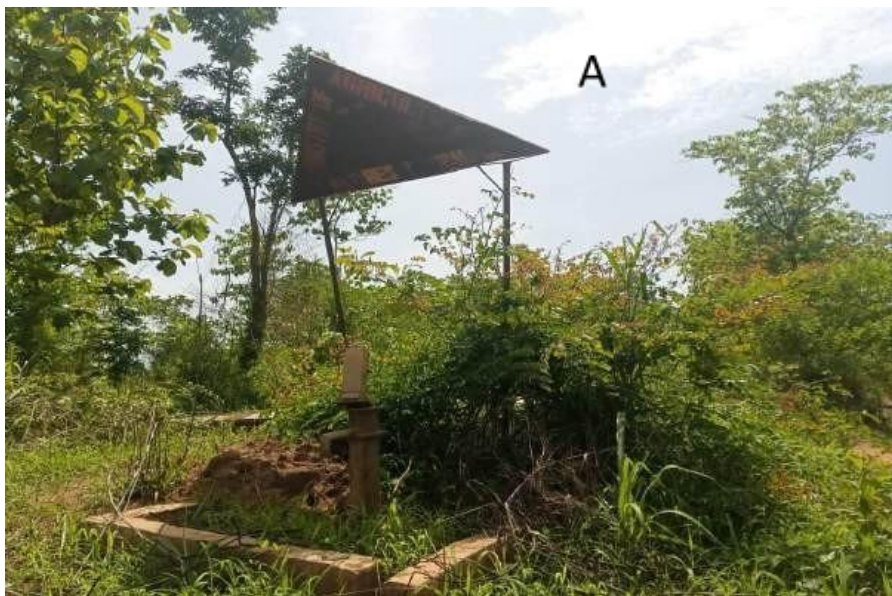
Plate 4.18a: Social infrastructures at proposed AIH site A – abandoned borehole, B - electric cables and wires without a transformer and C – fallen poles
